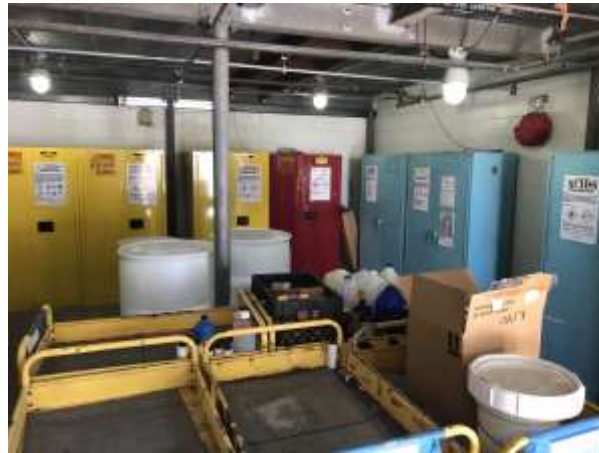
Photograph 20. Flammable materials cabinets in the Bulk Chemical/Hazardous Waste area.
