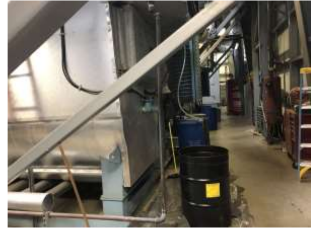
Photograph 27. View of the leak in the Chilling Room.
