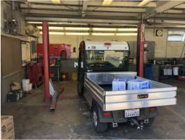
Photograph 1. View of the above ground lifts at the Facilities and Maintenance Auto Shop.
