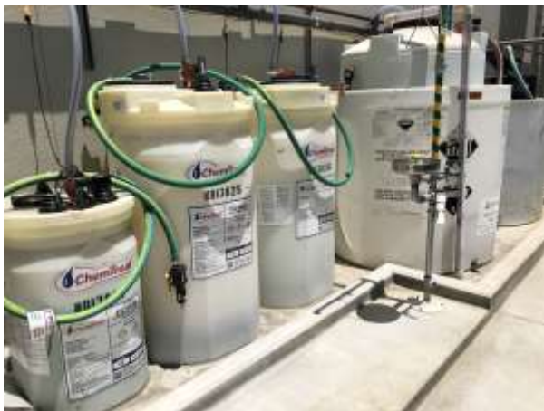
Photograph 28. View of bulk chemical storage outside the Chilling Room.
