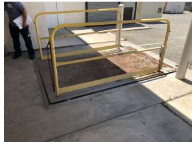
Photograph 30. Hydraulic lift at DHB loading dock.
