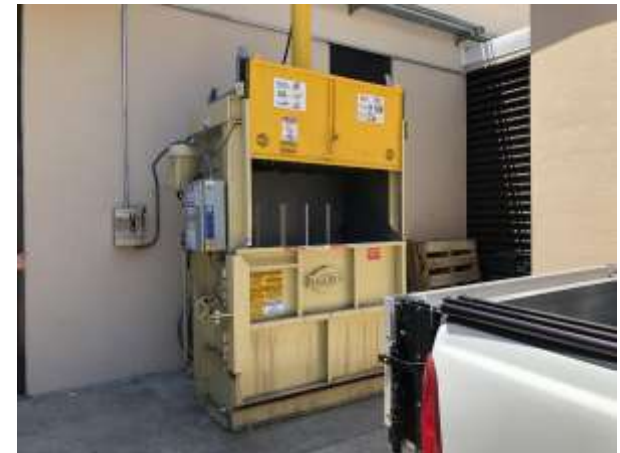
Photograph 12. View of the trash compactor north of the Titan Student Union loading dock.
