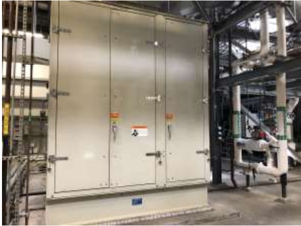
Photograph 25. View of one of the chillers in the Chilling Room.
