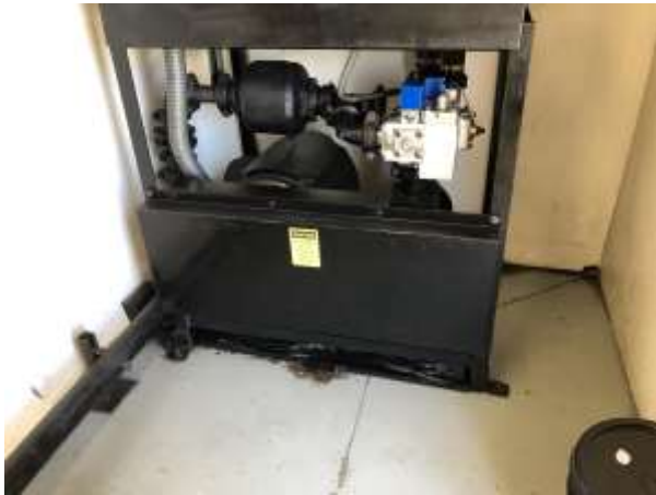
Photograph 31. View of the elevator equipment in the DBH building.
