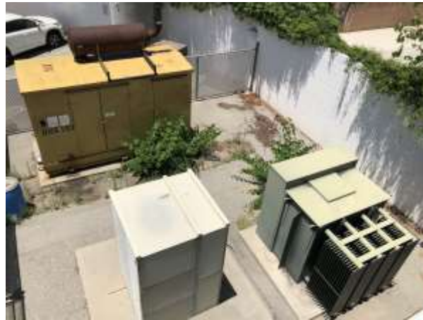
Photograph 32. View of the DBH generator and one reported leaking transformer.
