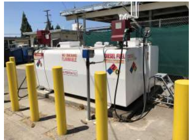
Photograph 6. View of the onsite 1,500-gallon diesel AST near the Receiving buildings.
