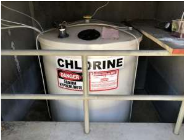
Photograph 10. View of the chlorine tank at the Student Rec Center.
