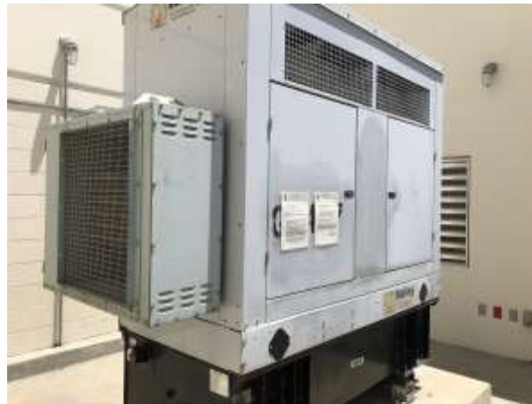
Photograph 11. Diesel fueled generator outside the Student Rec Center.
